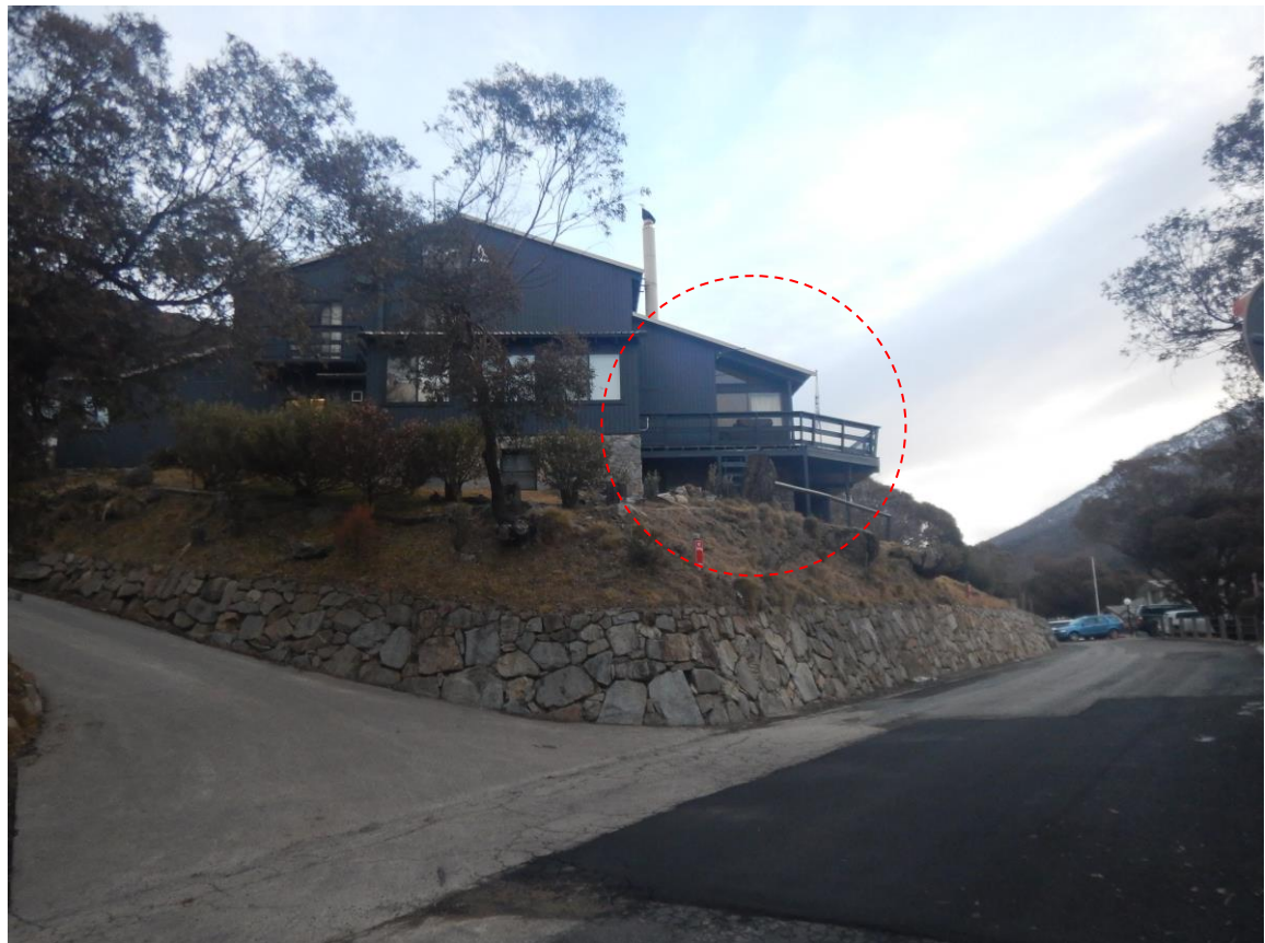
Figure 7: Photo of the north eastern elevation showing deck to be removed and wall to be extended
